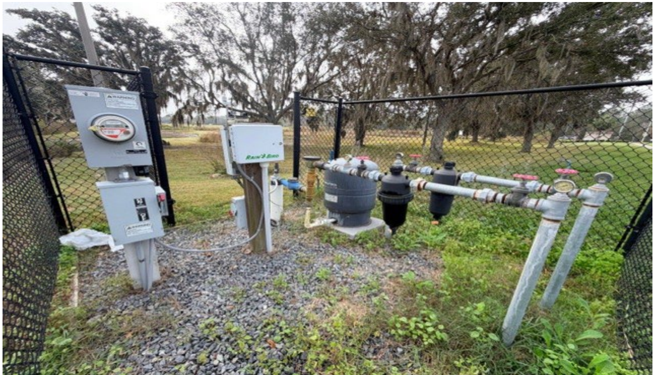
Figure 2: Photograph of the groundwater well DID No. 5 at Hidden Creek North. Photo taken January 7, 2026, by Edward M. Craig IV , CPSS of Ardurra Group, Inc.
