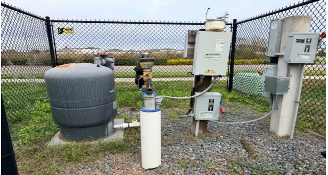
Figure 1: Photograph of the groundwater well DID No. 5 at Hidden Creek North. Photo taken January 7, 2026, by Edward M. Craig IV , CPSS of Ardurra Group, Inc.
